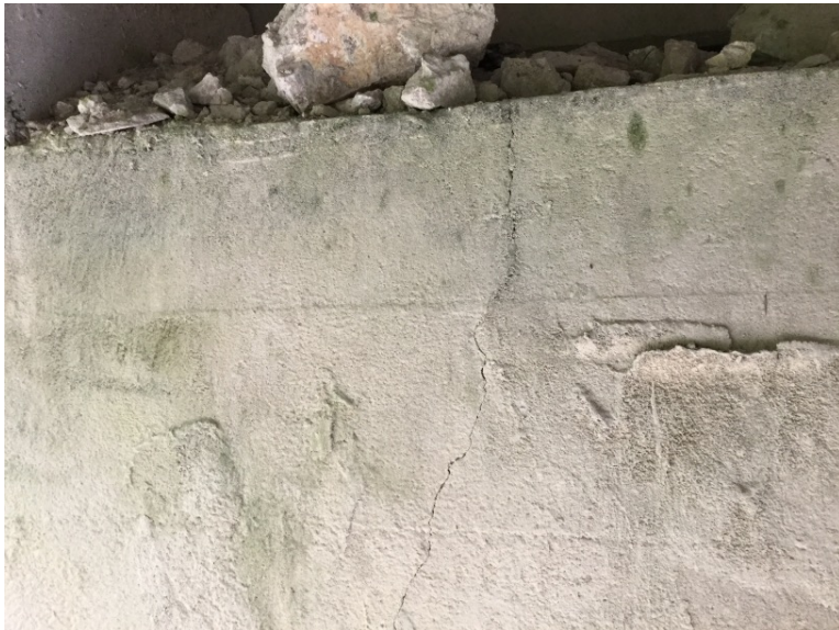
Vertical crack in CIP upstream left bank
